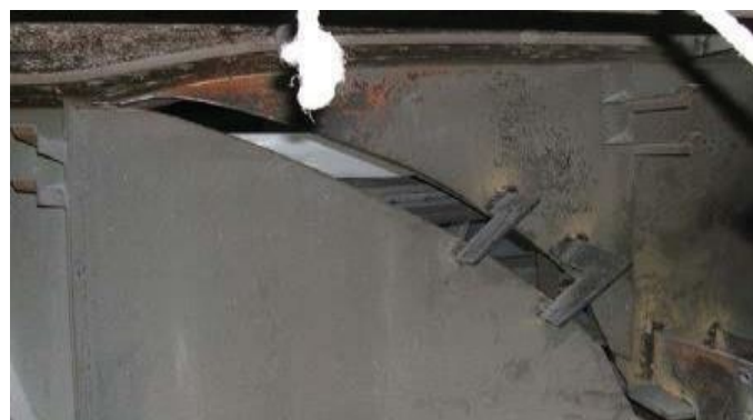
Figure 1. Actual crack of crane girder.
