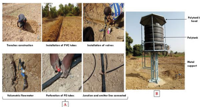
Figure 4. 4a) Installation of drip irrigation kits 4b) Presentation of the tower after its installation.
