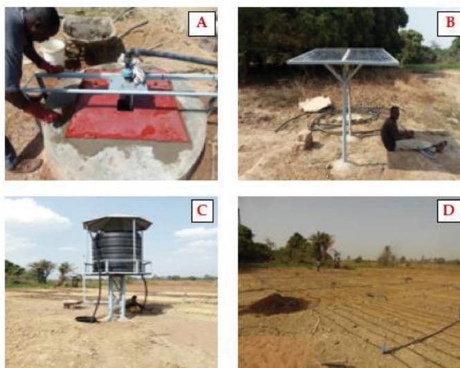
Figure 6. Different components of the drip irrigation system 6a) Solar pump immersed in the well 6b) Solar installation 6c) Water storage device 6d) Irrigation kit device.
