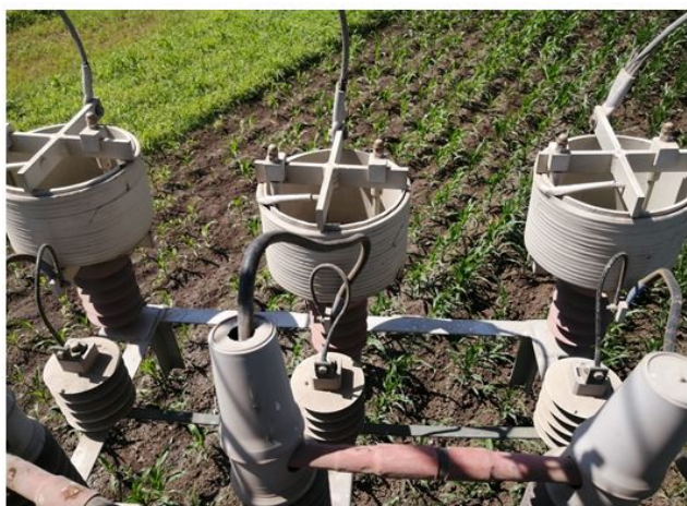
Figure 4. The old STPF at bus 10 at Elgendy distributor.
