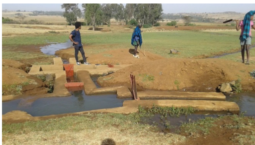
Figure 4. Ashar main canal division gates unable to control water loss.
