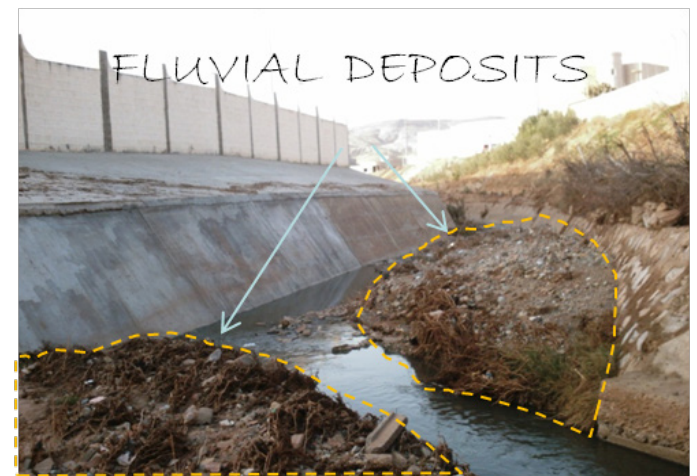
Figure 12. Alluvial deposits on the bottom of the channel.
