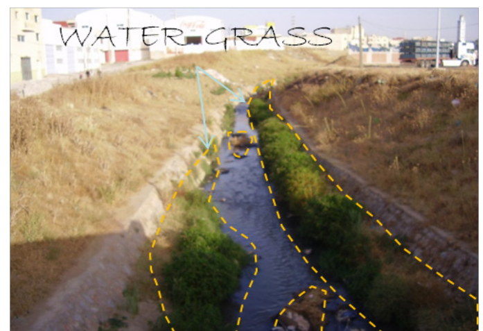
Figure 13. Water grass on the floor and edge of the channel.
