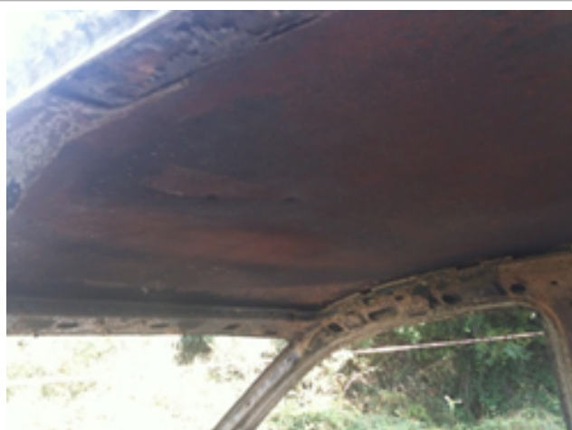
Figure 3: Two concave depressions in the metal sheet.
